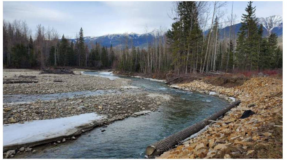
Nearly three million dollars is being invested to help protect the homes of residents living along the Dore River near McBride. The money will provide 1200 metres of large rocks- riprap along stretches of river bank that are particularly vulnerable to erosion during high water. /ANDREA ARNOLD
