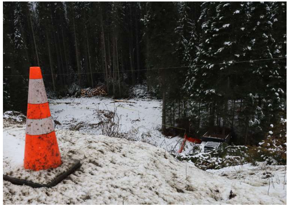
Soil removal operations at the Clemina crash site were underway the week of March 25th, according to the Ministry of Environment. Environmental consultants have been making regular trips there to assess the impact of the truck crash. / ABIGAIL POPPLE
